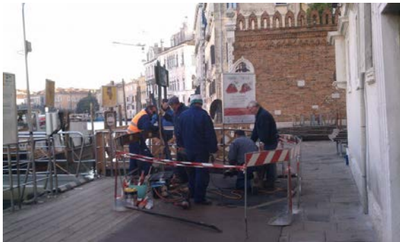
Figure 10: Construction produces high Noise Levels
